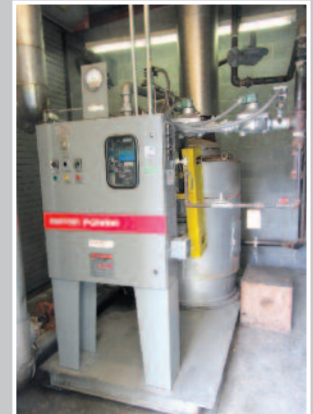
VAPOR Power Boiler
